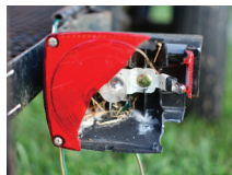
Damaged trailer lighting
